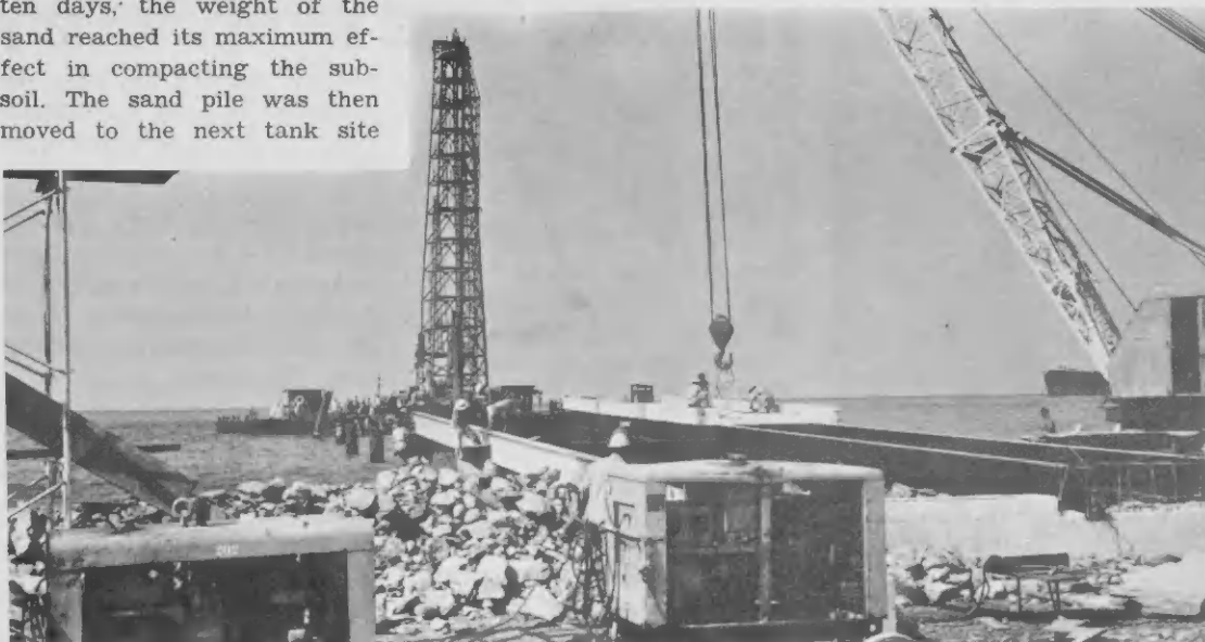
A "bridgehead" ashore is being built, while a pile driver is installing piles for a trestle to a 60 by 80 feet platform being 500 meters from shore for Lago's Offshore berth.
